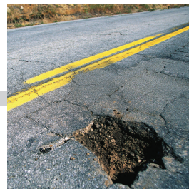
POTHoles/ DAMAGED PAVEMENT
