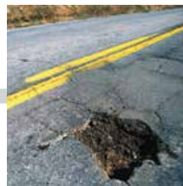
POTHoles/ DAMAGED PAVEMENT
