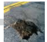
POTHOLES/ DAMAGED PAVEMENT
