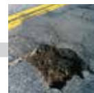
POTHoles/ DAMAGED PAVEMENT
