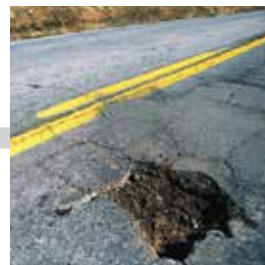
POTHOLES/ DAMAGED PAVEMENT
